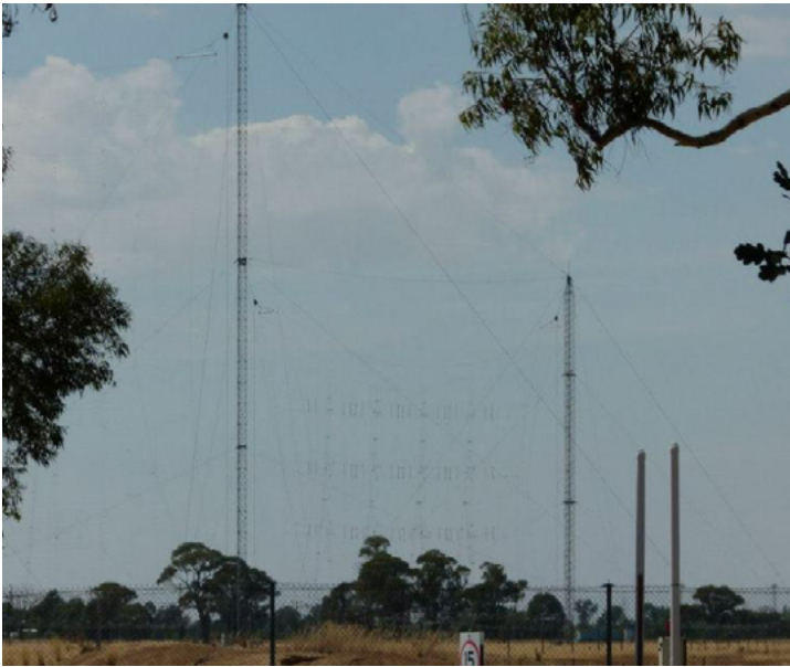
Former Radio Australia shortwave transmitting antenna at Shepparton, Australia (Courtesy: Radio Australia)
