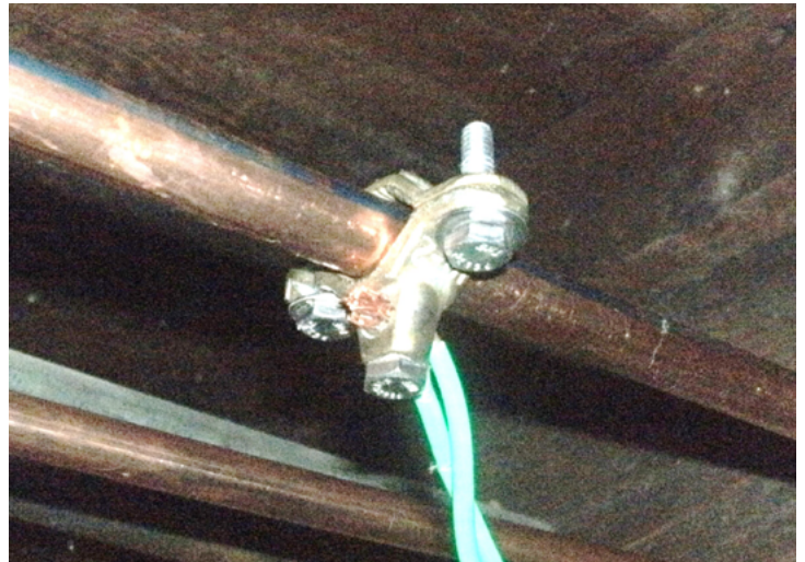
Safety ground near the author's operating position. NOT a good RF ground. (Author's photo)
